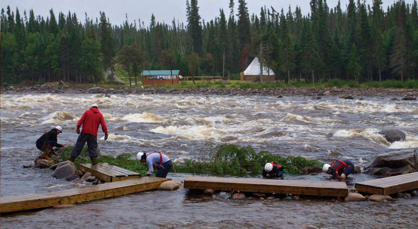
Downstream scooping weir in construction on the north shore of Smokey Hill
